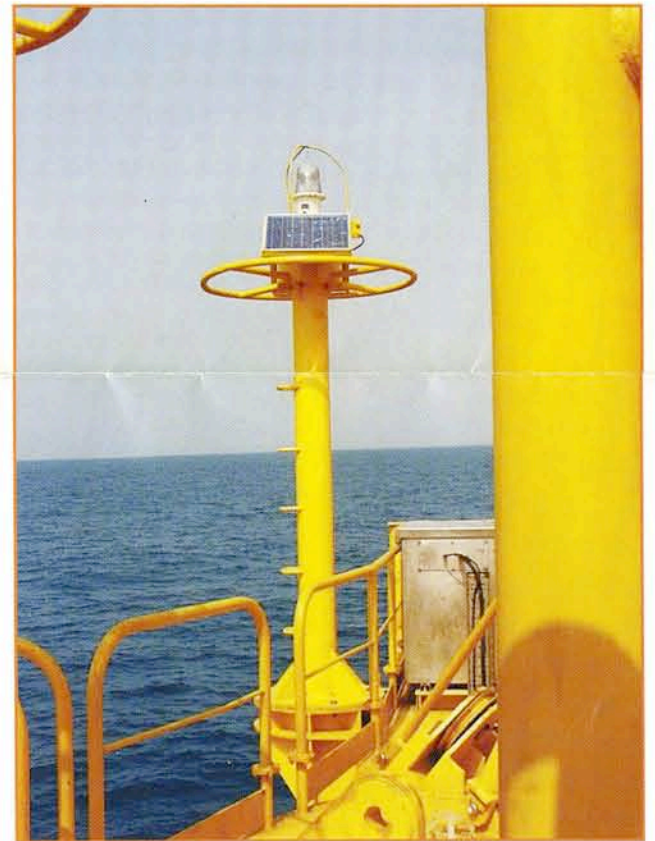
Resinex signalling pipes installed on SBM monobuoy
